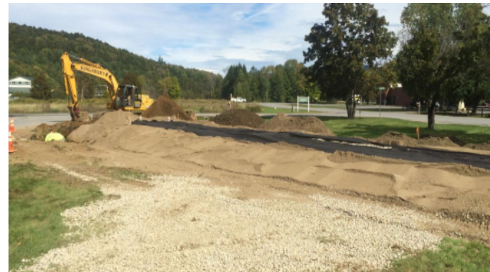
Construction of Mound Wastewater Disposal Area for Irasville Business Park in Waitsfield, VT
