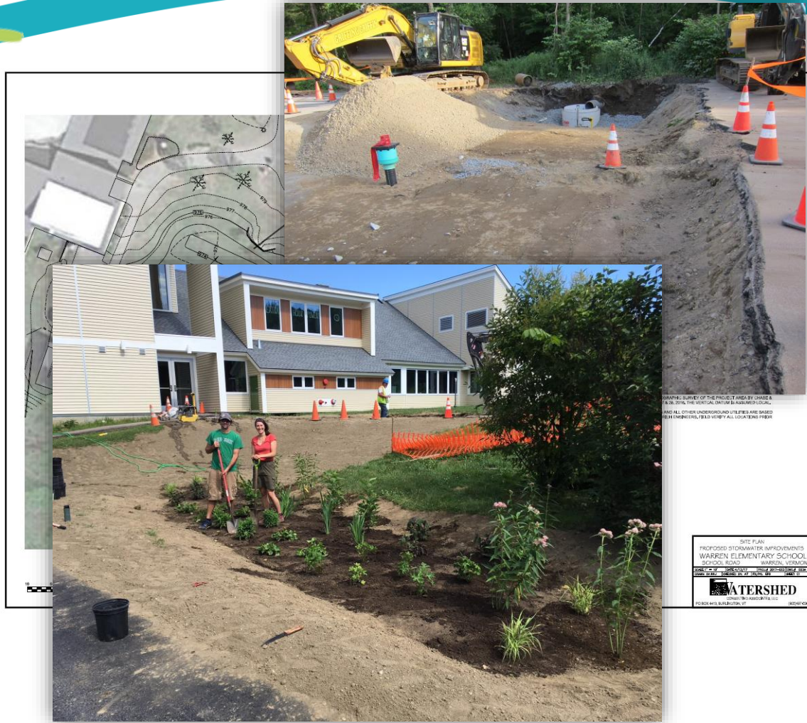
Warren School SWMP, sub-surface chambers, & raingarden
