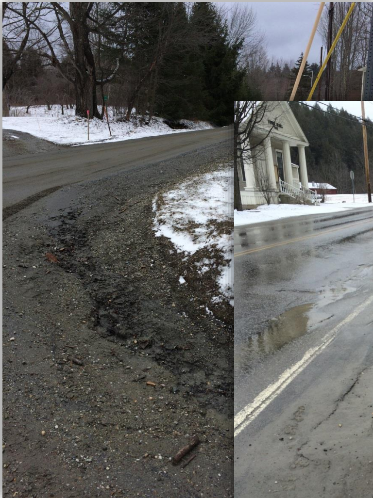
Runoff Causes Maintenance Issues
