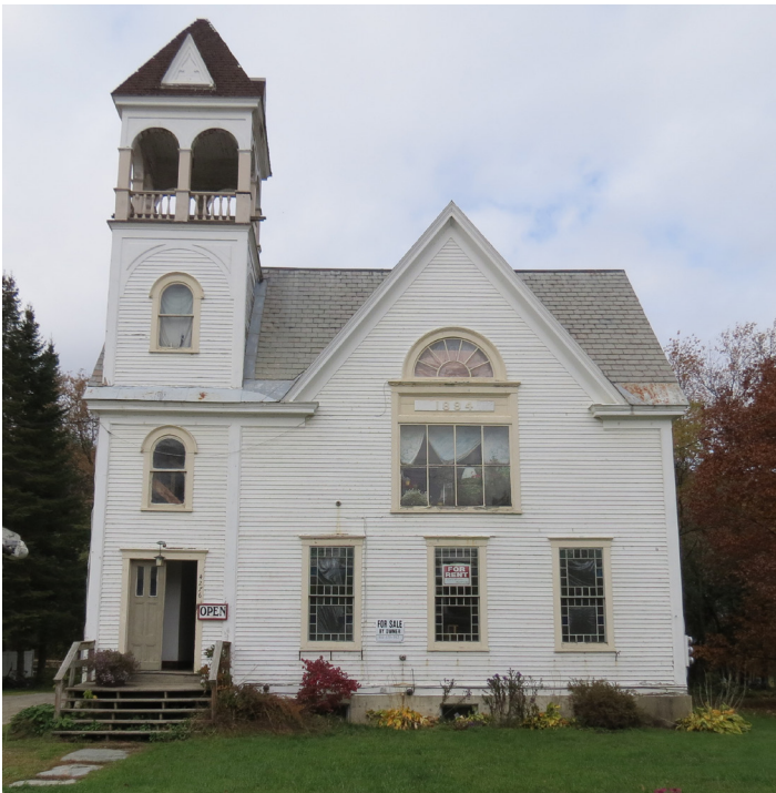
4276 Vermont 100 – Existing Façade Conditions
