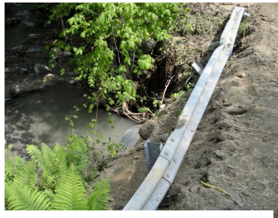
Eroded culvert due to stormwater, Mad River Valley
