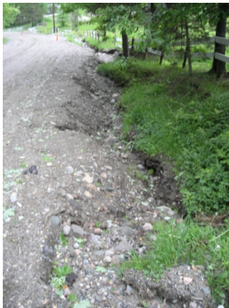
Roadway eroded after May 2011 storms, Mad River Valley
