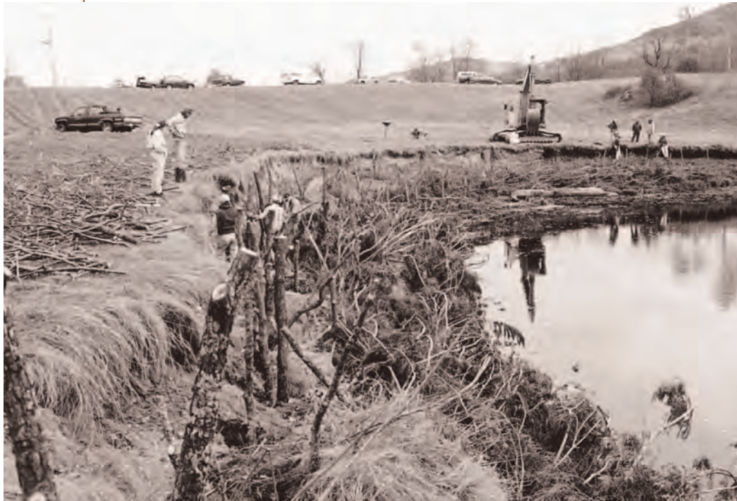
Volunteers install a streambank stabilization system on the banks of the Mad River, Fall 1996.
